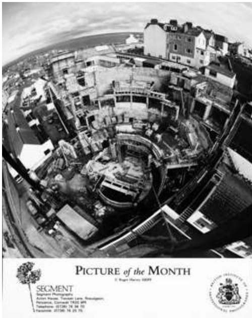
Figure 85. Photograph showing an aerial view of the construction site of Tate St Ives. The Gallery was built on the site of a derelict gasworks overlooking Porthmeor Beach. (Tate Archives)
