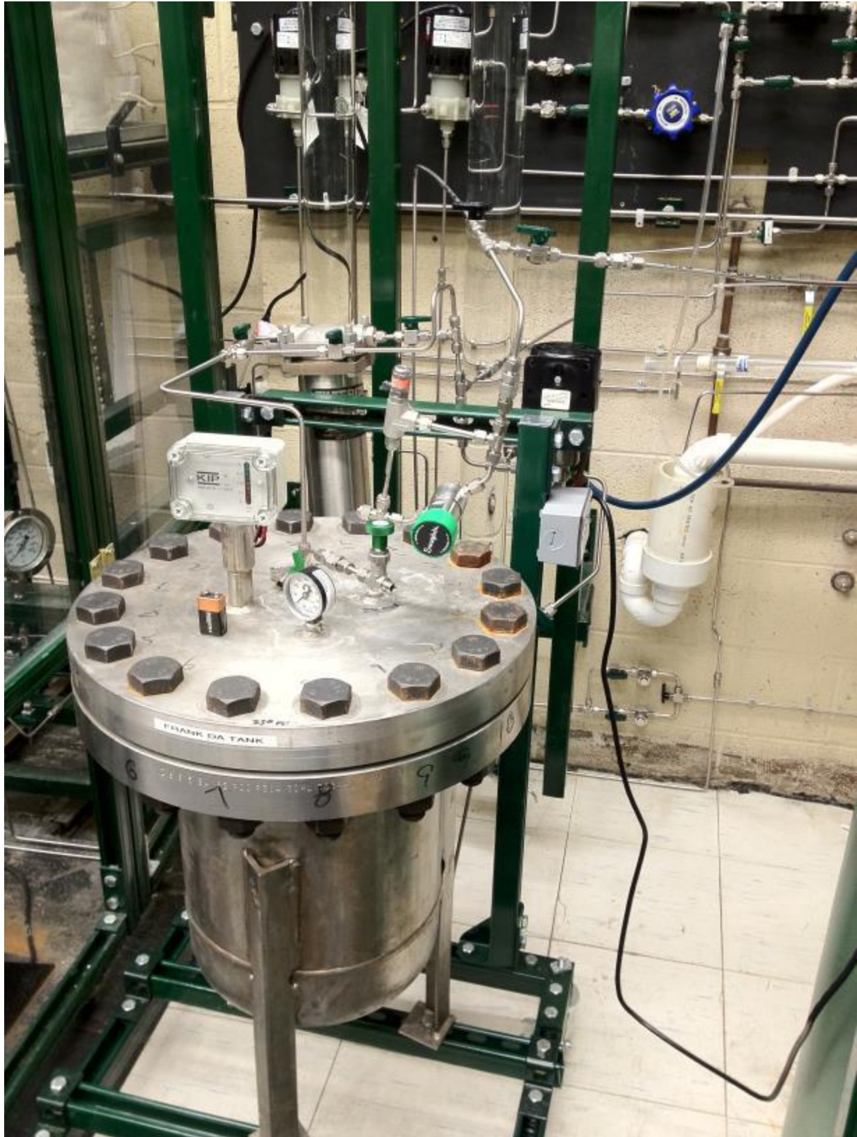
Figure 3.6. Feed water (Frank da) tank.
