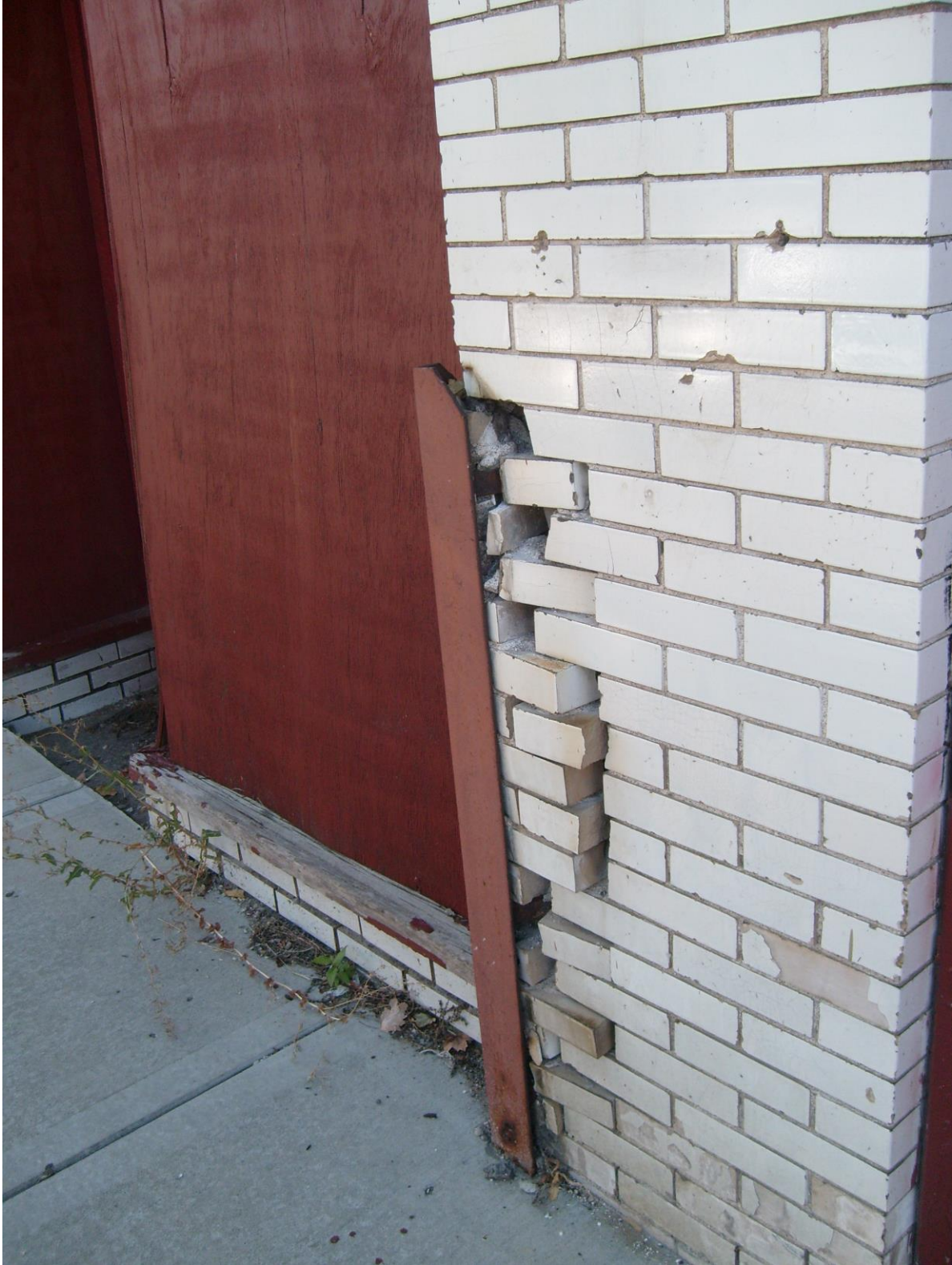
Figure 3.22: Façade exteriors on Vine street are in most places literally falling apart (Photo taken by author).
