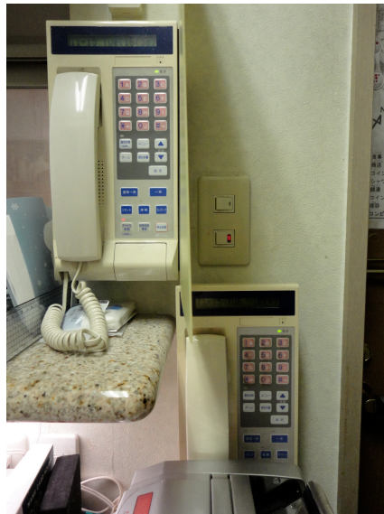
Figure 17. A Nurse Call System Installed at Mr. Okamoto's Office
