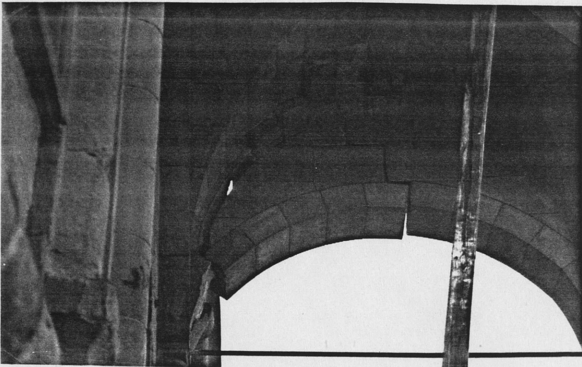
(b) Loose stones in arch
