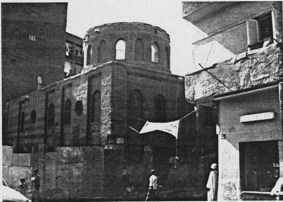
Fig. 11 Collapsed dome of El-Dashtwati Mosque
