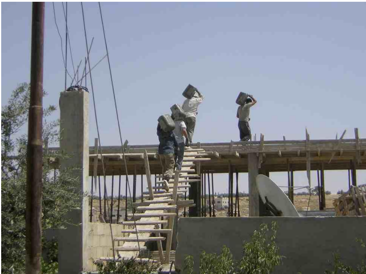
Figure 3: Workmen are laying the roof of the apartment. It would eventually consist of a 4x4 meter kitchen (on the left) and a 4x4 meter room on the right with a 2x2 meter hallway and a 2x2 meter bathroom. During the second phase, Harun's family added three more rooms in front.
