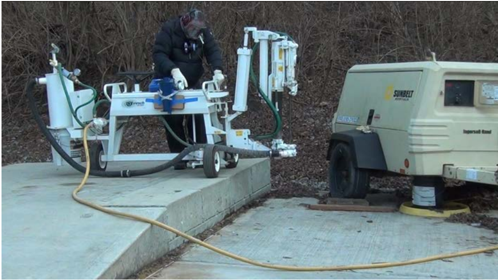
Figure 4.1 Proximity of the drill operator to the dowel drill and the air compressor
