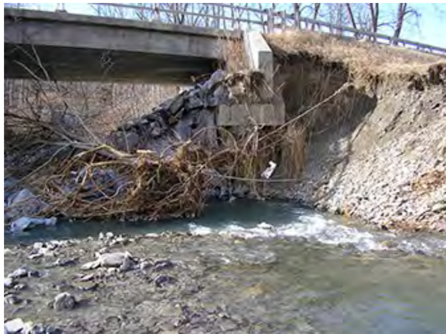
Structural damage caused by erosion. (Source: US Department of Transportation Federal Highway Administration)
