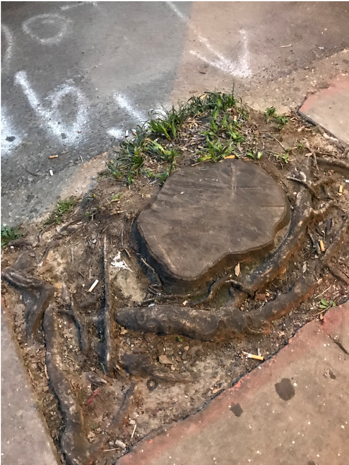
Figure 4.3b. With the tree removed, but the stump still visible, tree root penetration pattern into the sidewalk appears evident.
