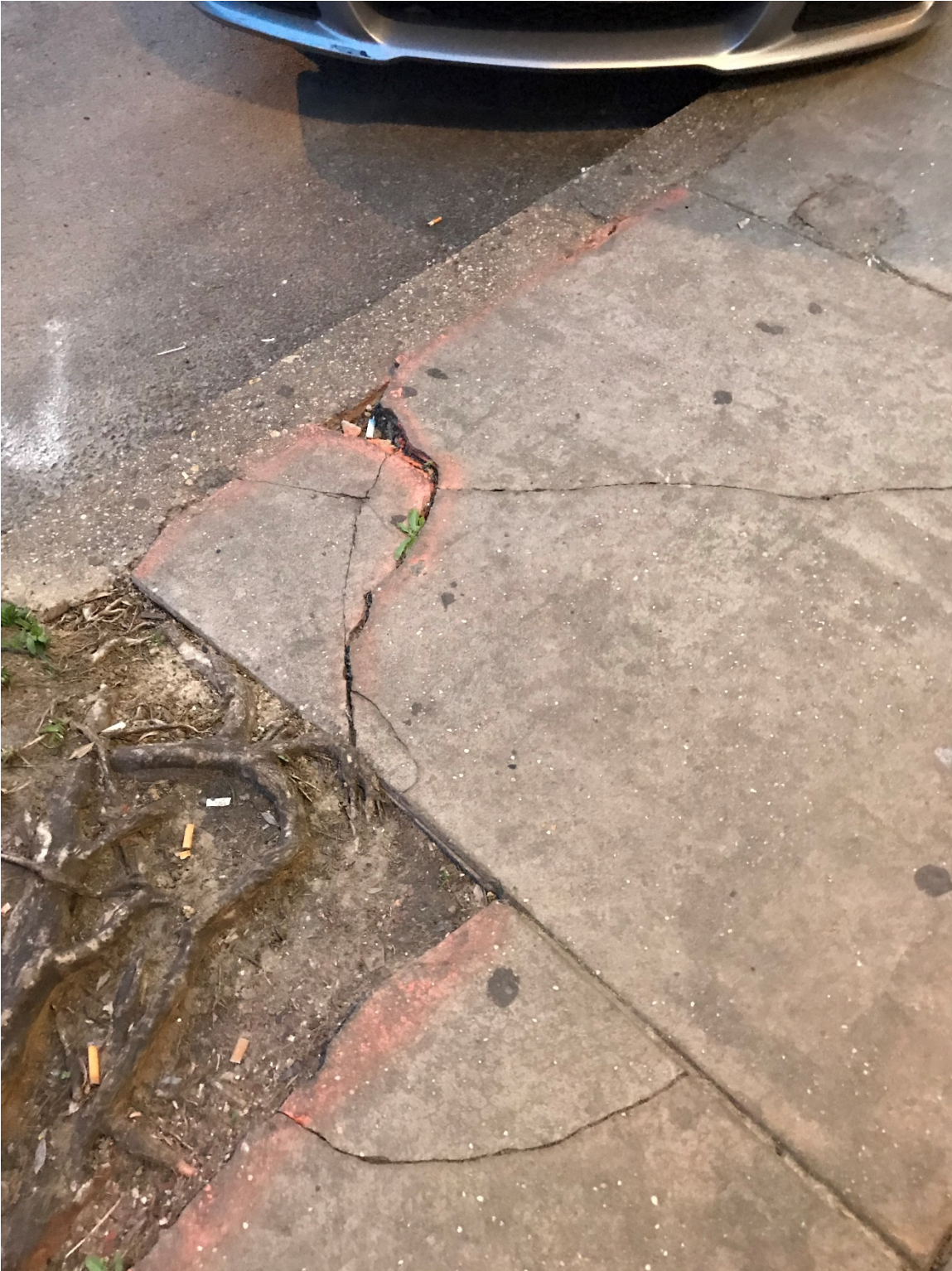
Figure 4.3a. Viewed from the street, the parked car blocks the view of sidewalk damage apparently caused by tree roots.
