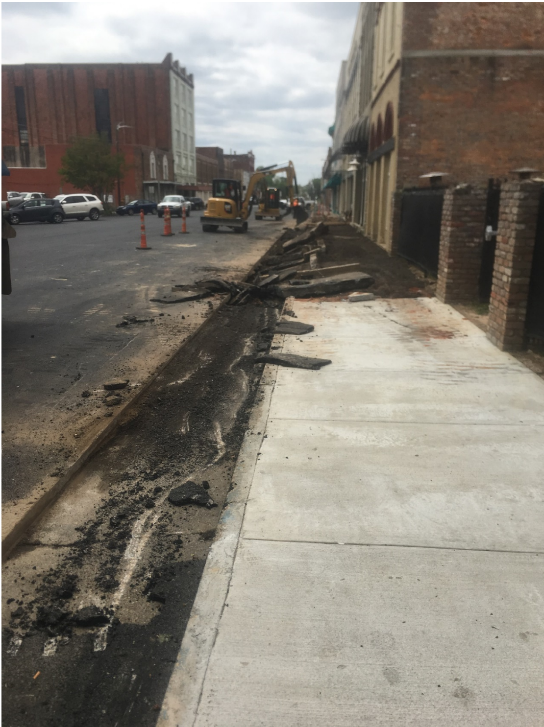
Figure 4.5. Front Street sidewalk, April 9, 2018. The new sidewalk in front of the Brickhaus Courtyard remains. All else was removed.
