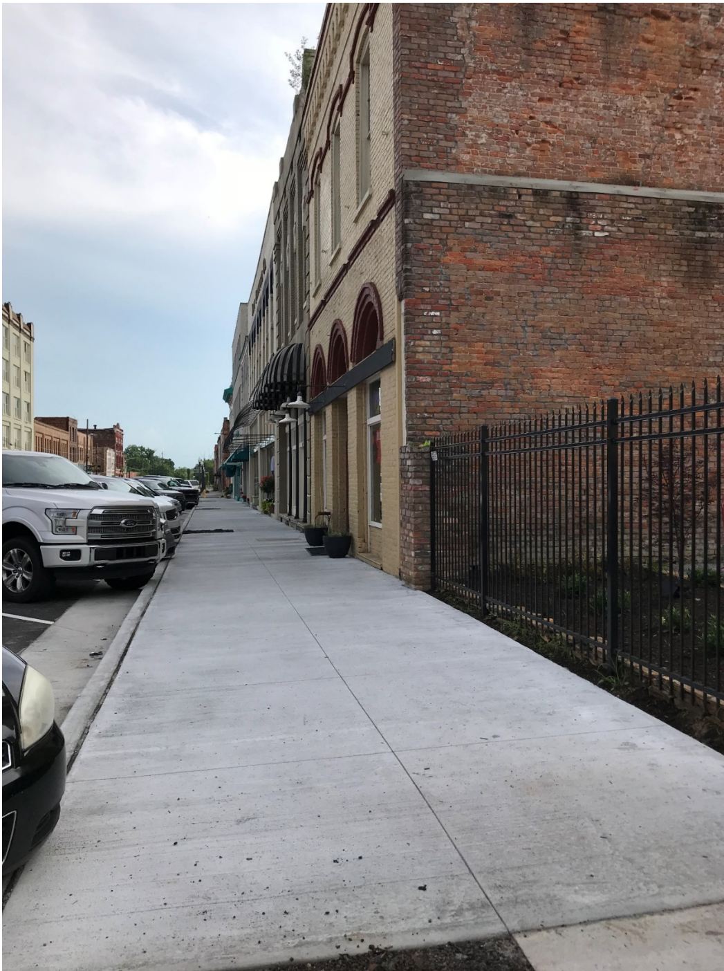
Figure 4.6. May 22, 2018. New sidewalk, curb, gutters, street, and parking in place. Lights and plantings to come.
