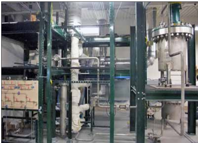
Fluoride test facility (Sun)
