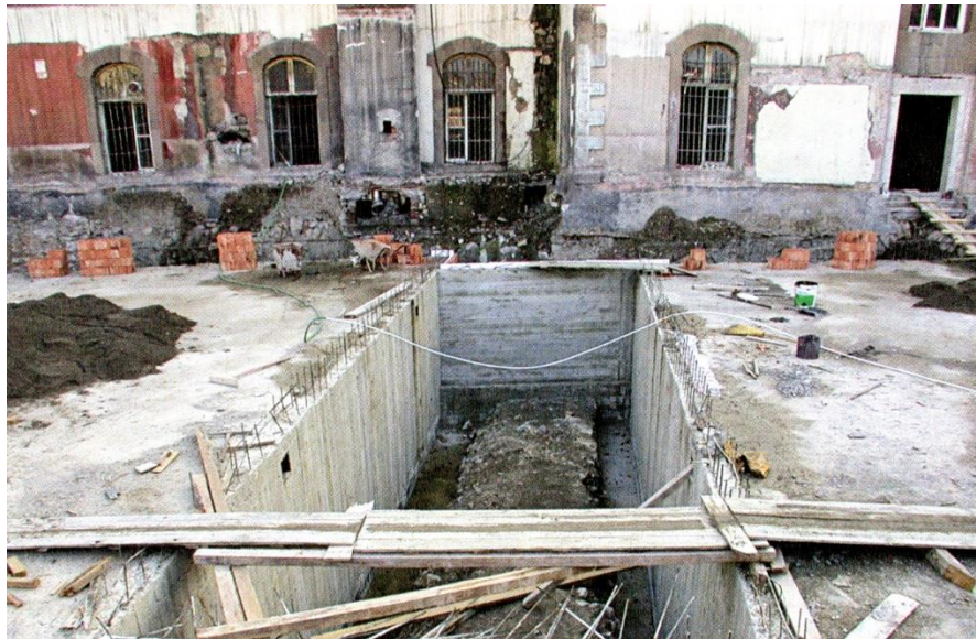
Figure 3.14. New boiler room, constructed on top of the Cardo Maximus . (After Kadioğlu Görkay Mitchell 2011, p. 150, fig. 81).
