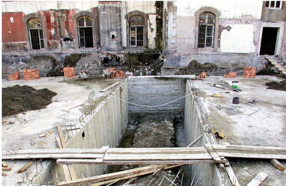
Figure 3.50. Remains of the Cardo during the excavation of the boiler room. (After Kadioğlu Görkay Mitchell 2011., p. 150, fig. 81).
