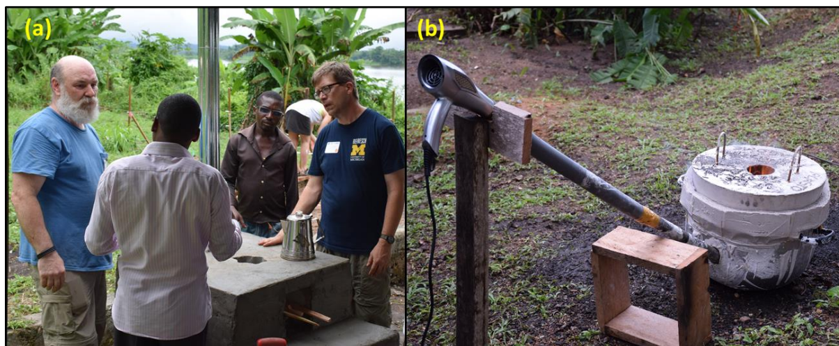
Figure 3.13 (a) A completed cookstove constructed on-site using locally available materials under demonstration (b) An aluminum smelter with an air-flow duct constructed on-site at Lambaréné
