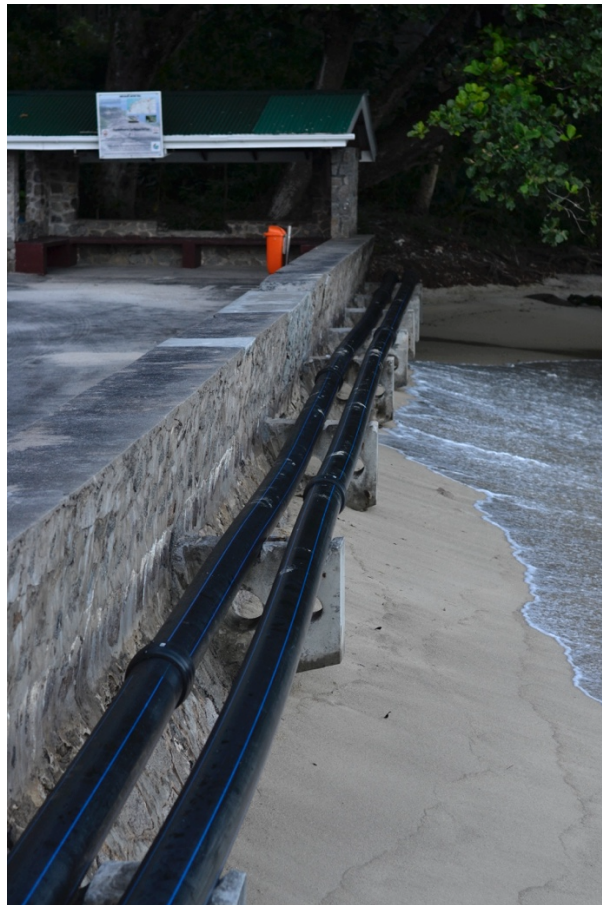
Figure 2.4: Exposed pipes adjacent to Bel Ombre Road
