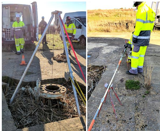
Fig. 3.10. Image of brine well (left) and wireline cable (right) used for field testing.
