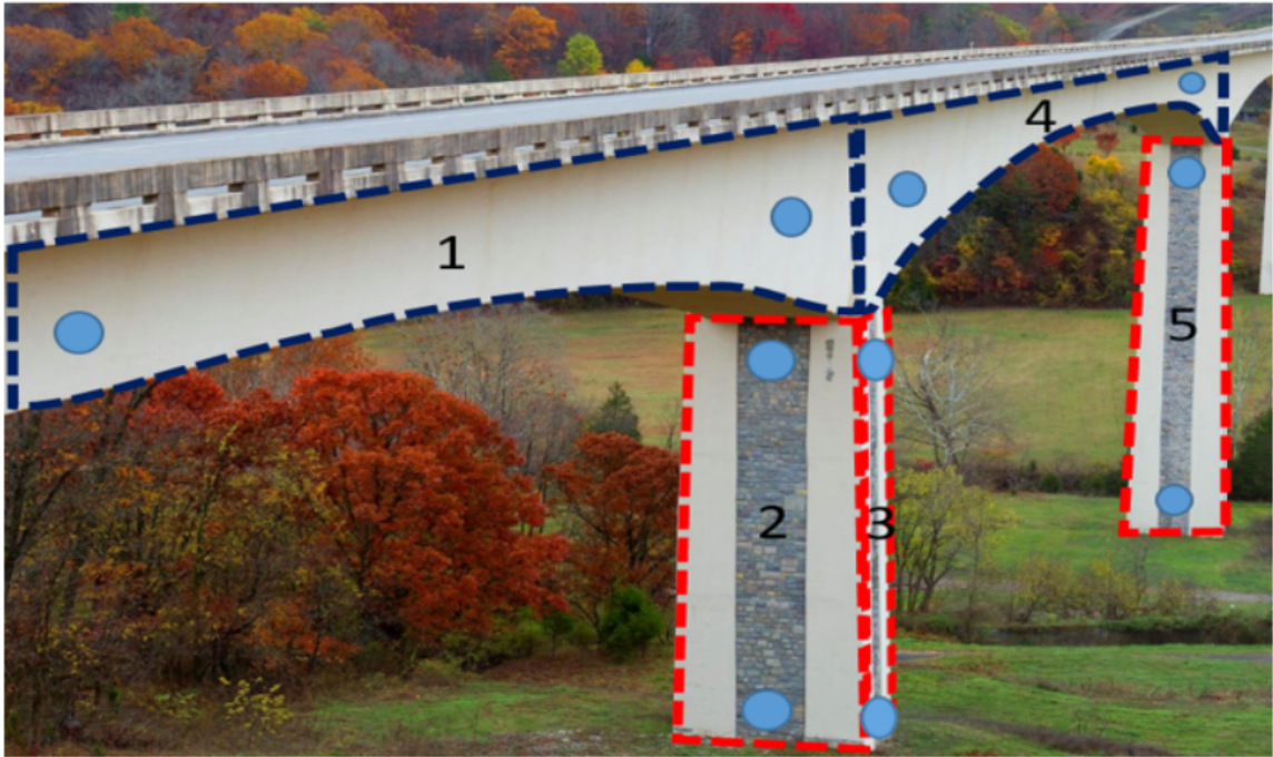
Figure 1.2: The authors of [3] reduce the number of waypoints required for bridge structural inspection by partitioning the bridge into a set of surfaces with entry and exit nodes. The high level sequencing of surfaces is accomplished with a Traveling Salesman approach while the low level observation of surfaces is accomplished with a local coverage controller.
