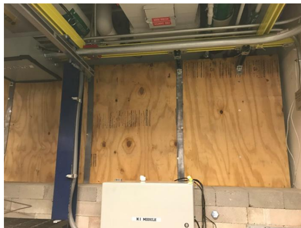
Figure 2.38 Concrete blocks and lead-lined plywood panels for the X-ray radiography system
