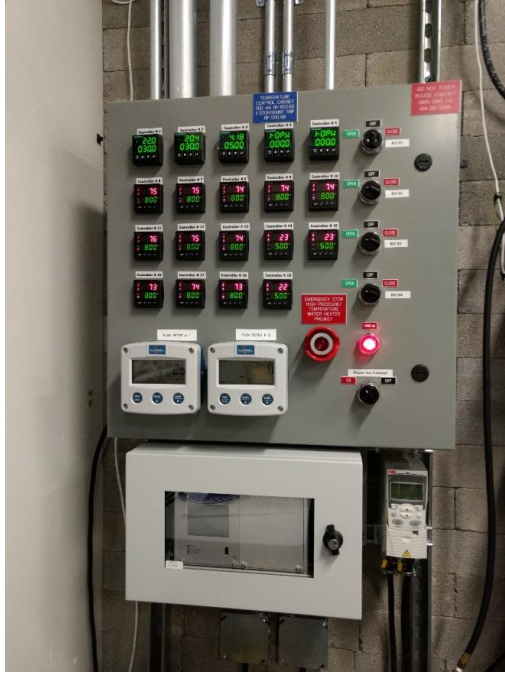
(a) Control panel: Temperature controllers et al.
