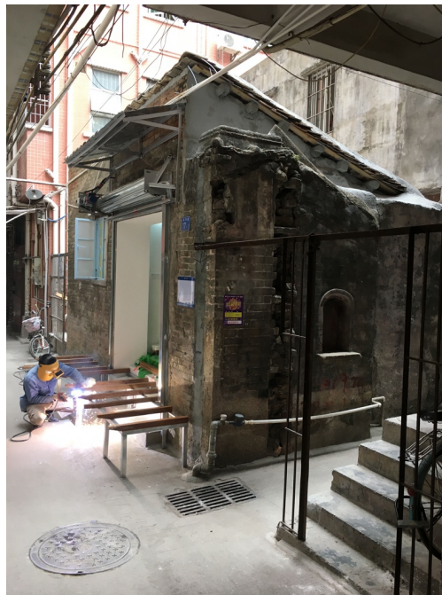
Figure 5-1. A migrant contractor working on an old house as a renovation project for the 2017 UABB at Nantou
