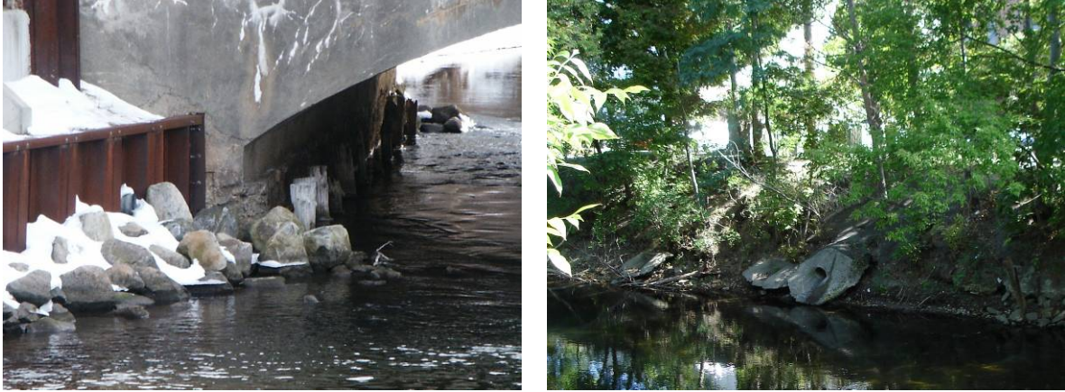
Figs 65a,b: A retaining wall on the south side of the Boardman River, A stormwater outfall on the Boardman River
