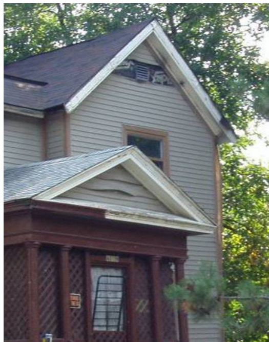
Figure 4.1: The neighborhood could benefit from some exterior repairs on this home.
