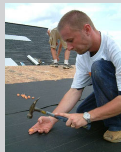
Figure 4.2: Volunteers can be very effective at repairing and painting existing homes. Source: Rebuilding Together website
