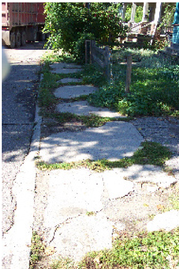
Figure 6.8: Many sidewalks in the neighborhood have been damaged during demolition or suffer from lack of maintenance.
