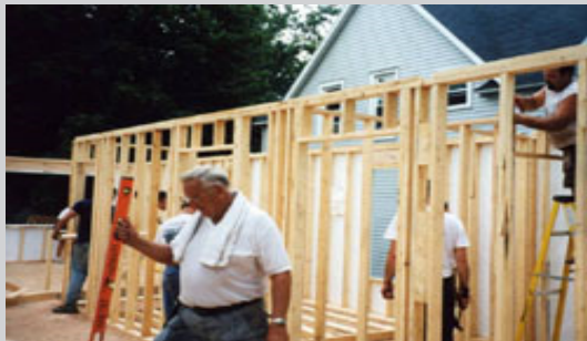
Figure 5.3. Construction in Kent County, Michigan, using "sweat equity". Source: Habitat for Humanity Kent County.
