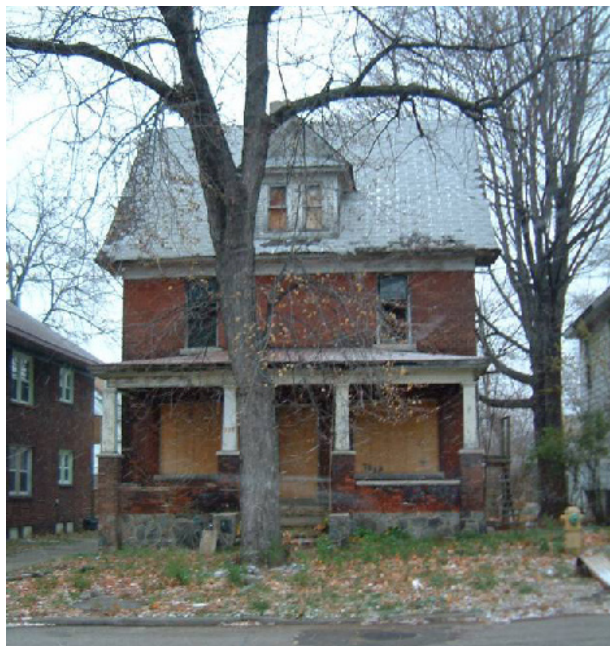
Figure 4.8: Although on a side street (Oak Street), this house is visible to all traffic heading into downtown on Fifth Street. Rehabilitation or demolition of this property would have a positive impact on the neighborhood appearance and image.
