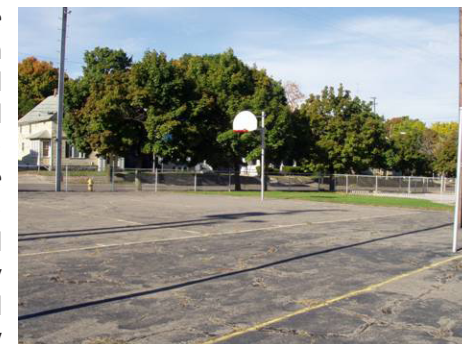
Figure 7.6: The basketball court in Memorial Park is in need of repair.
