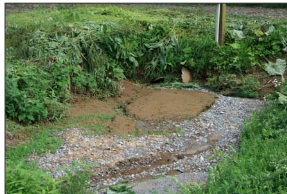
Figure 19: Erosion associated with a makeshift culvert near the farm complex
