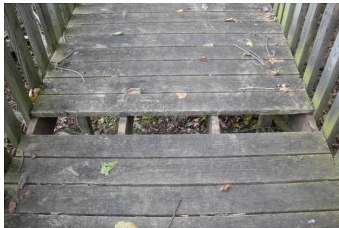
Figure 3.7: Missing board on one of the OEA bridges. (Photo by Rebecca Gajewski)
