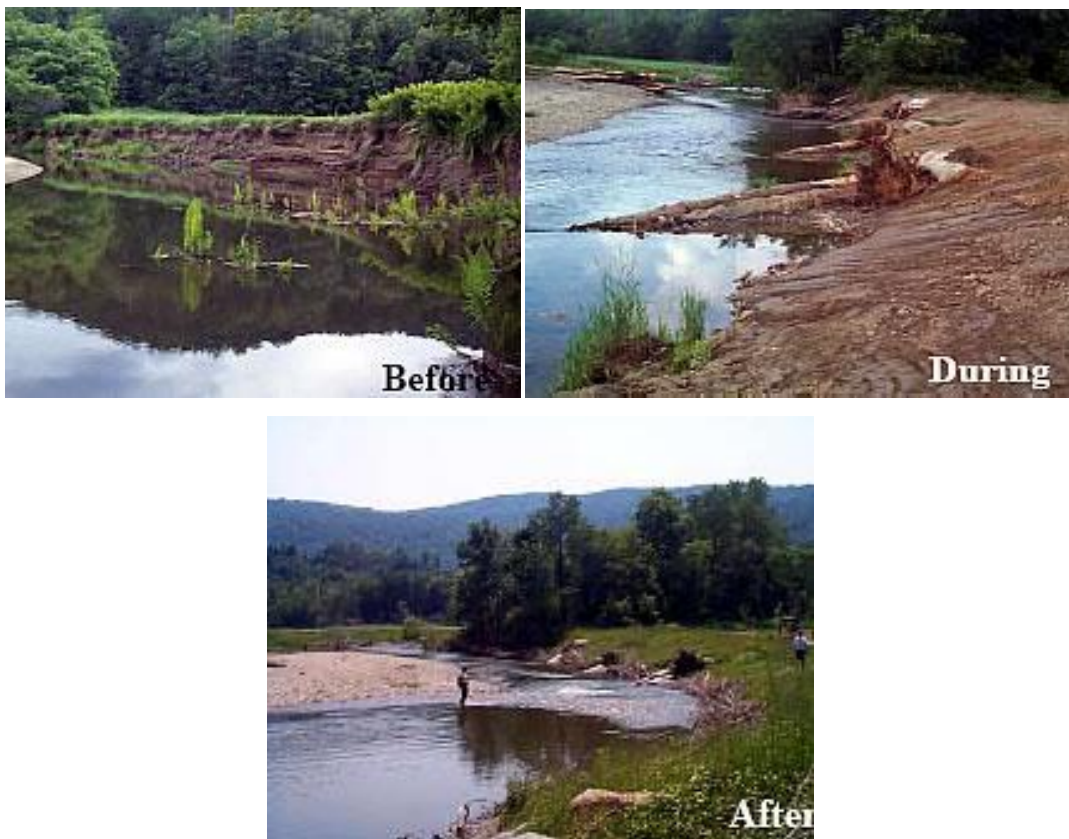
Figure 1.9: Example of river corridor restoration involving reducing the height and forming more gradually sloping streambanks. These actions, taken by Vermont’s Agency of Natural Resources (ANR) and River Management Program, helped to stabilize this stream’s banks and reduce deposition of sediments and phosphorus into the stream. (Photos by Vermont Clean & Clear Plan: Agency of Natural Resources: http://www.anr.state.vt.us/cleanandclear/rivstrm.htm )
