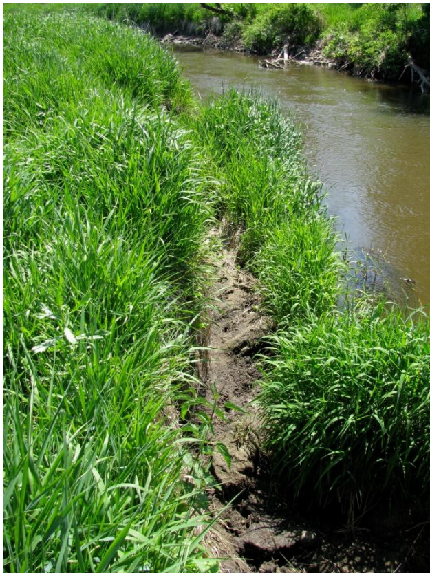
Figure 1.8: Streambank erosion on Mill Creek within the Village's proposed Mill Creek Park that is causing sections of the bank to begin slumping into the stream. (Photo by James Minesky)
