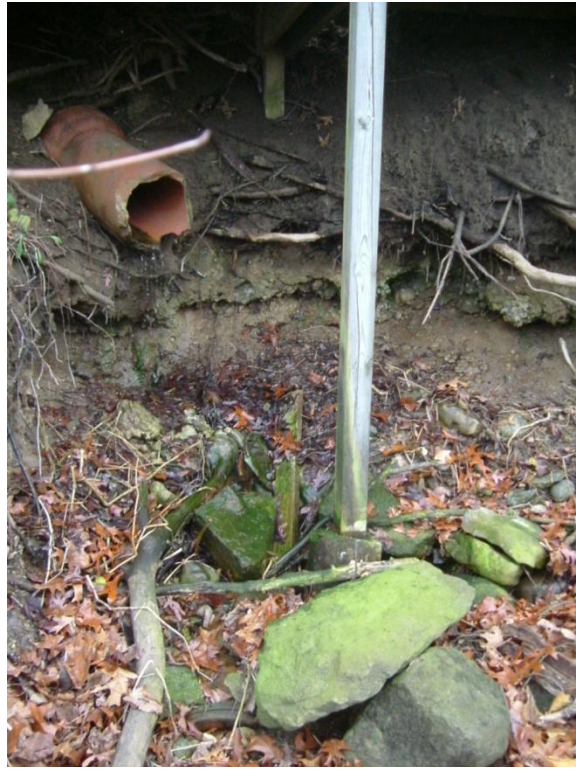
Figure 2.5: Outfall C-1 and critical support beam for above wooden bridge. (Photo by Patrick Reed)
