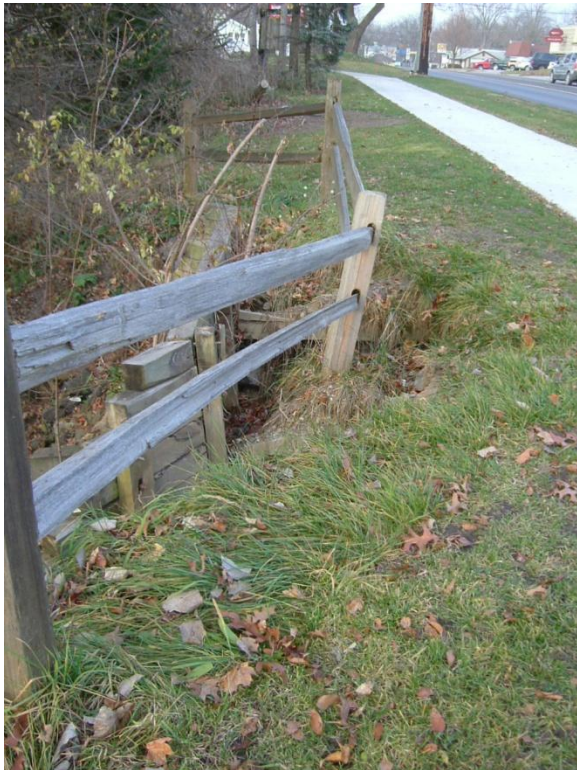
Figure 2.4: Erosion around the Baker Road outfall moving toward the sidewalk. (Photo by Patrick Reed)
