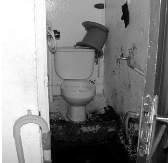
Figure 8.6 Home-made improvements to SIDR Petite Ile bathroom
