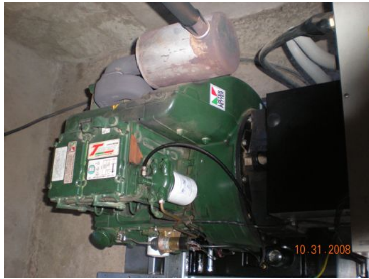
Figure D.5: Petrol Generator at MPALA
