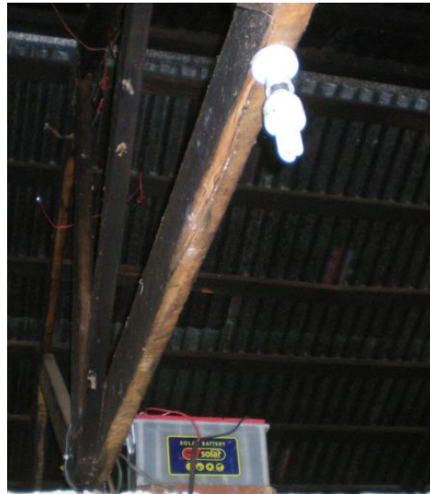
Figure 3.11: A battery system connected directly to a CFL
