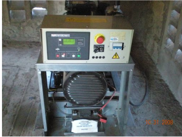
Figure D.4: Diesel Generator at MPALA
