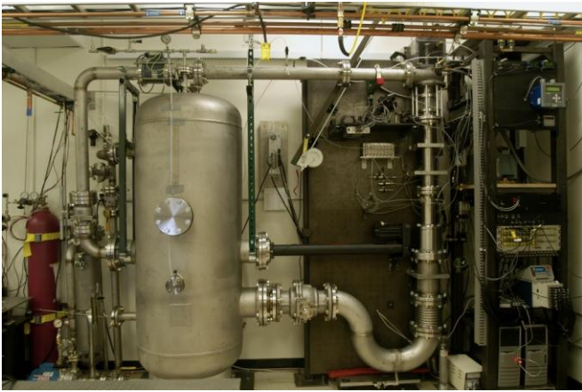
Figure 3: Cavitation Test Facility
