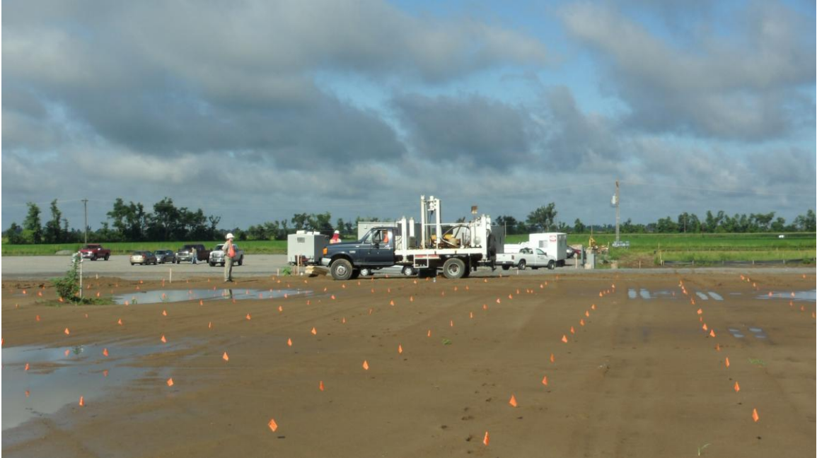
Figure 6-1. Construction site at New Madrid, MO with flags showing impact pier installation points (photo courtesy of Russell Green).
