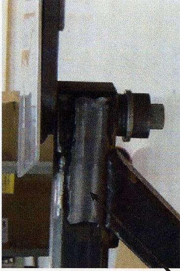
1/8 " steel plate used to reinforce weld between the arm joint block and truss structure (used on both sides of upper swing arm)
