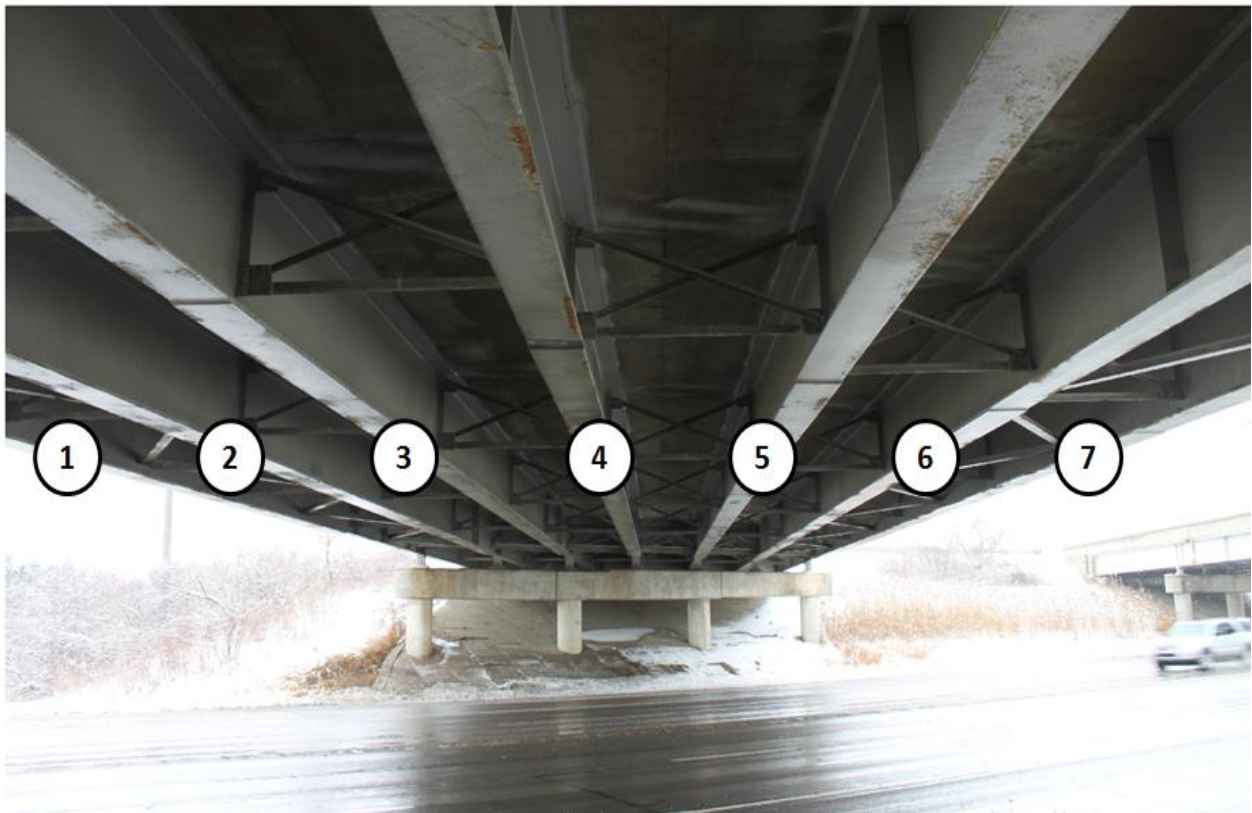
Figure 7.26: Underside of the CSB deck and the 7 girders that form the composite action system
