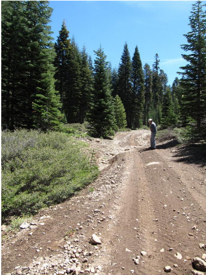
Picture 4: Washout on the Stanislaus National Forest.
