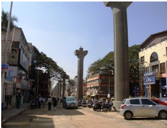
Picture 4.15. Metro pillars along CMH Road, Indiranagar. The space between the pillars are used for parking vehicles
