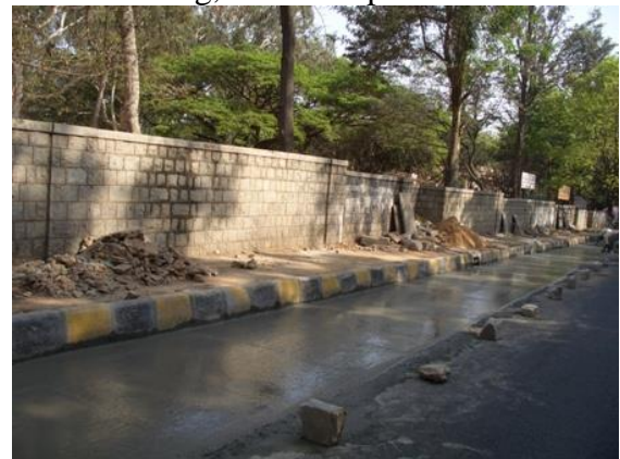
Picture 5.10. A freshly laid stretch of road for which the adjacent sidewalk was narrowed, Malleswaram
