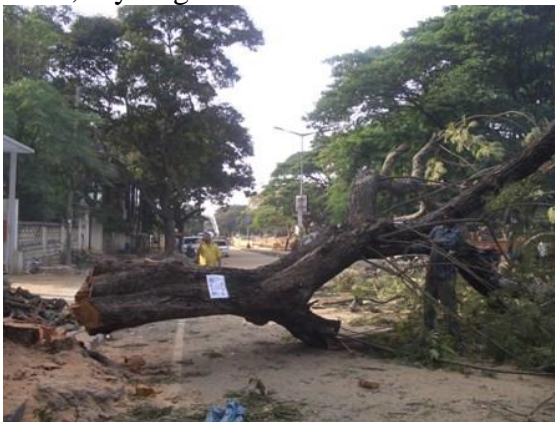
Picture 5.9. Tree felling at Tagore Circle to make space for constructing an underpass
