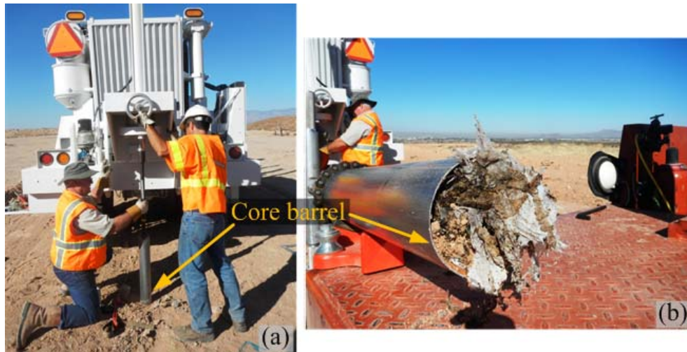
Figure 4.7 (a) Pushing core barrel to the waste mass and (b) recovered solid waste in the core barrel.
