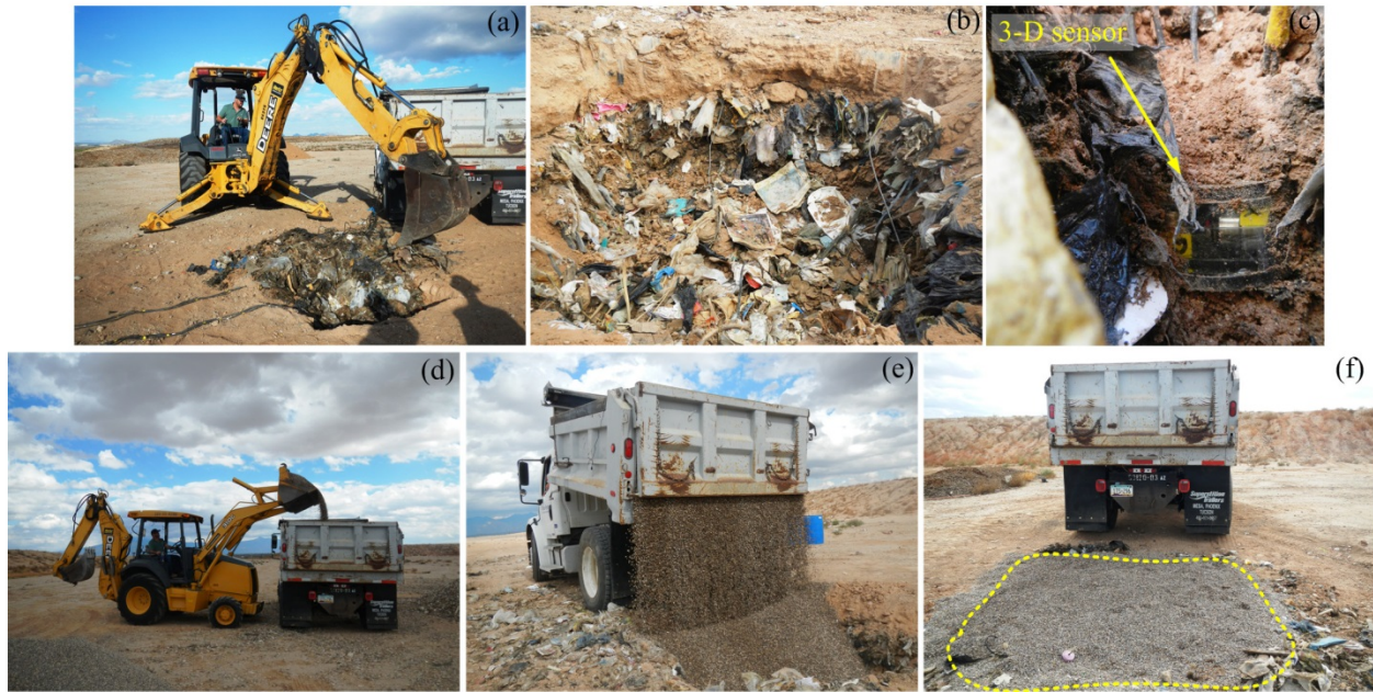
Figure 7.13 (a) Waste excavation, (b) MSW pit, (c) exposed 3-D geophone, (d) placement of gravel into truck, and (e and f) in-situ unit weight measurement at the LRL.
