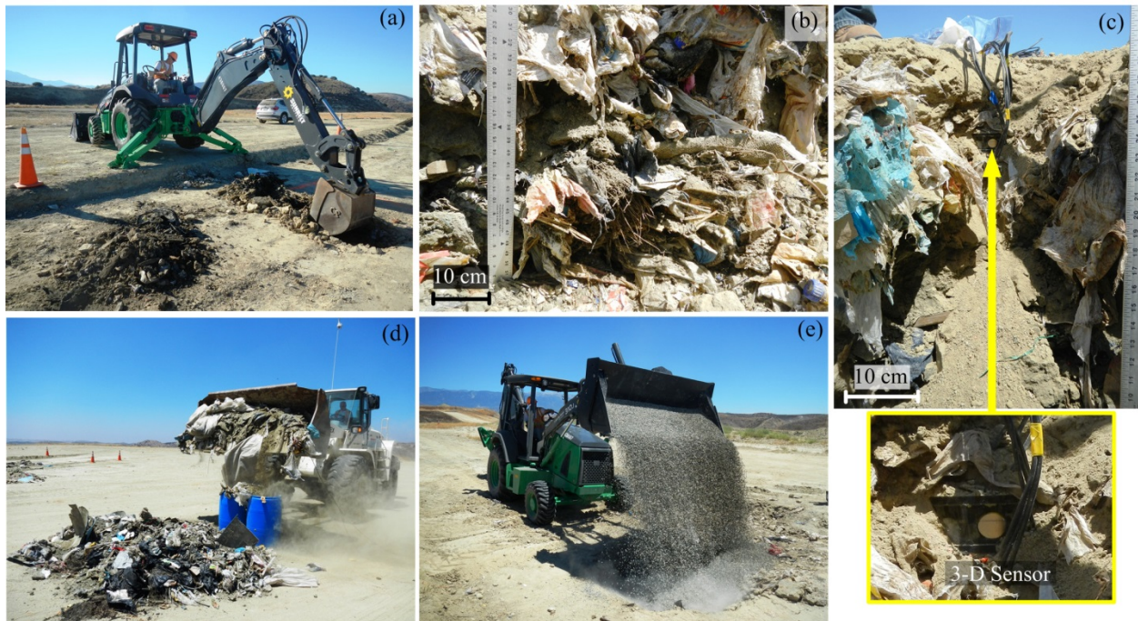
Figure 6.13 (a) Waste excavation, (b) MSW pit, (c) exposed 3-D geophone, (d) placement of MSW into drums, and (e) in-situ unit weight measurement at the LCSL.
