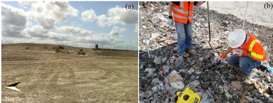
Figure 5.3 (a) Site view and (b) layer with large-waste-particle in location 1 at the ACL.
