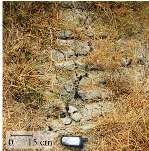
Figure 8.13 Soil cover cracks at the BKK.
