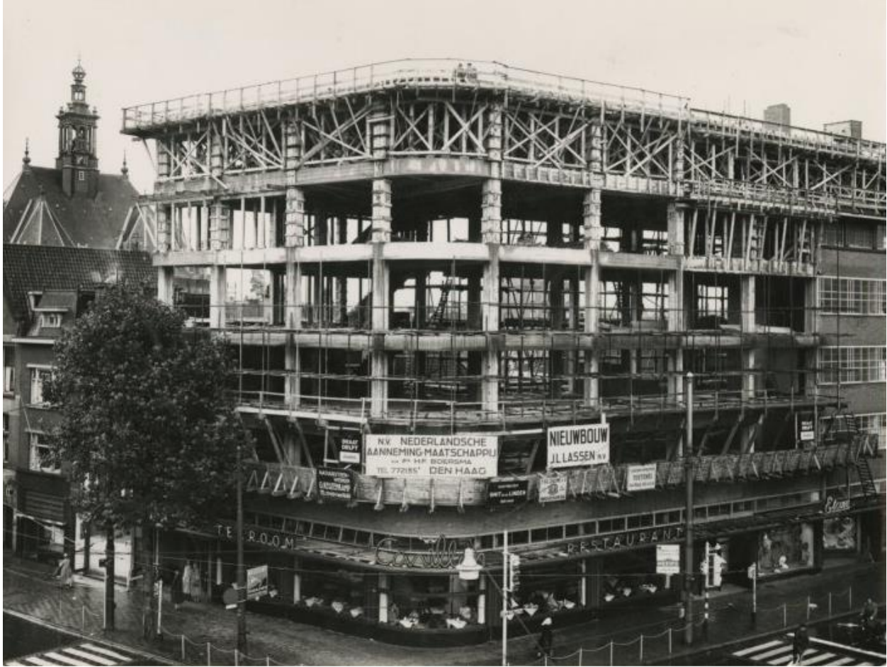
Figure 244. New construction for the Carillon lunch room, which was opened during construction. 1041
