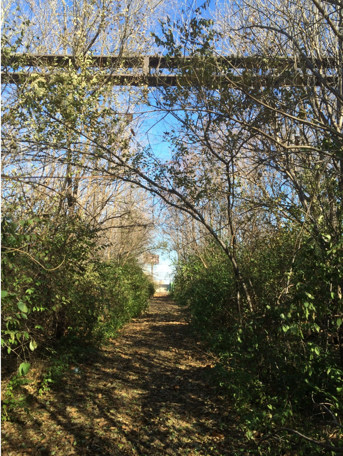
FIGURE 33: WESTERN END OF THE TRESTLE WITH GATE IN DISTANCE. PHOTO BY AUTHOR 2012.
