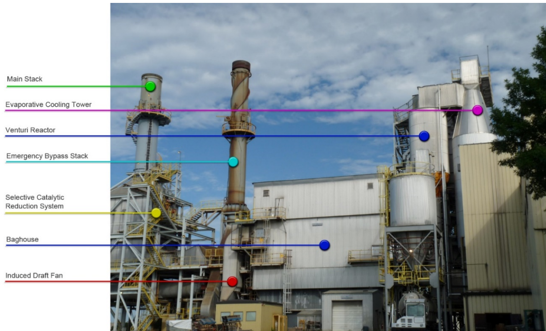
Figure 2. Photograph of the Emerald Energy from Waste facility [2].
