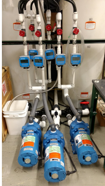
Figure 2.9: Components of the RCCS facility: Three centrifugal pumps, six flow monitors, and six flow control valves.
