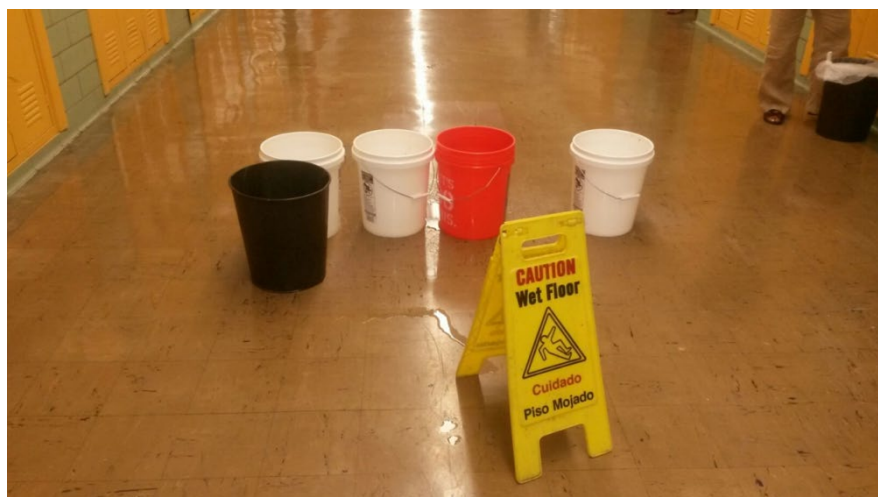
Figure 2: Cody MCH collecting ceiling leaks using buckets in the middle of school hallway where students travel between class and visit their lockers. Taken from the B. et al v Snyder et al Complaint, p. 94.
