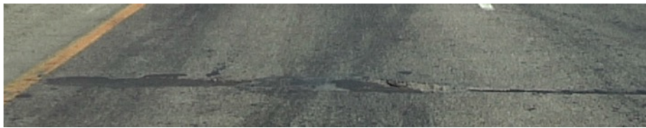
Figure 2.5 Image, deteriorated bridge joint
