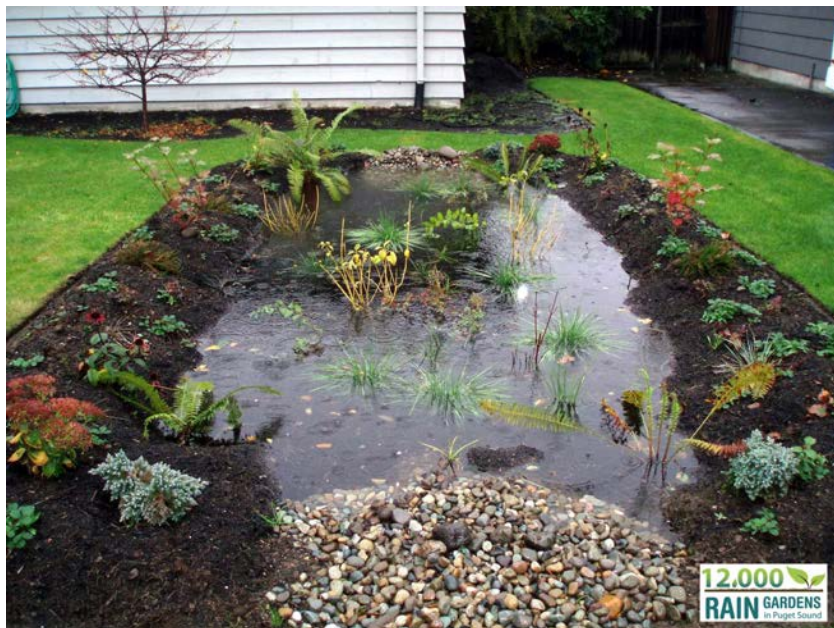
Figure 7. Typical rain garden construction with planted depression to store and infiltrate stormwater from nearby impervious surfaces (Williams, 2016).
