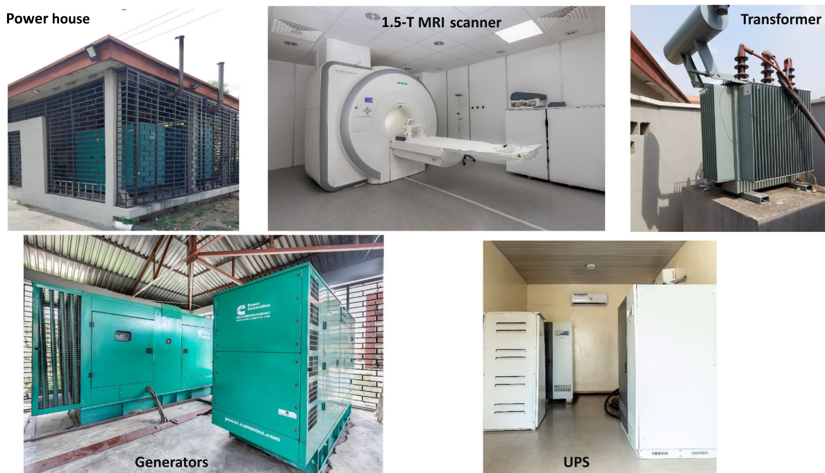
FIGURE 6 Energy solutions for steady power supply in SSA medical imaging facilities. Images of the local energy solution at Crestview Radiology Limited in Lagos, Nigeria, for steady power supply for operation of the MRI equipment and other imaging devices. MRI, magnetic resonance imaging; SSA, Sub-Saharan Africa; UPS, uninterruptible power supply
