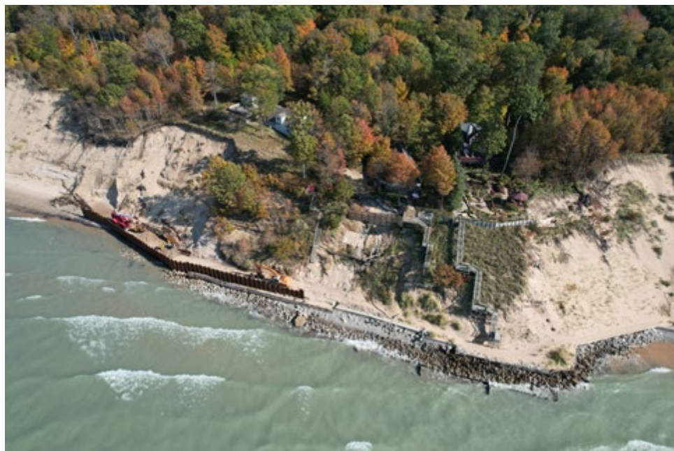
Figure 15. Active construction of a seawall along the Syndicate dune portion of the lakeshore observed in June of 2022.
