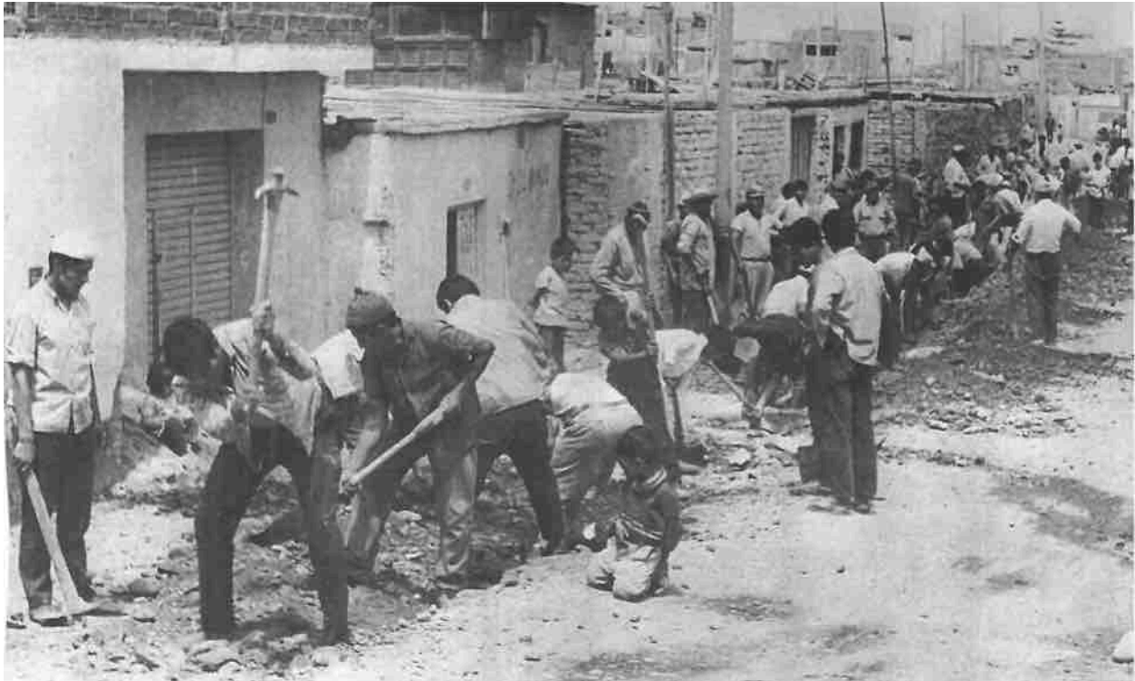
Plate 3.1. Men participate in a collective works project to install a neighborhood sewage line, ca. 1956
