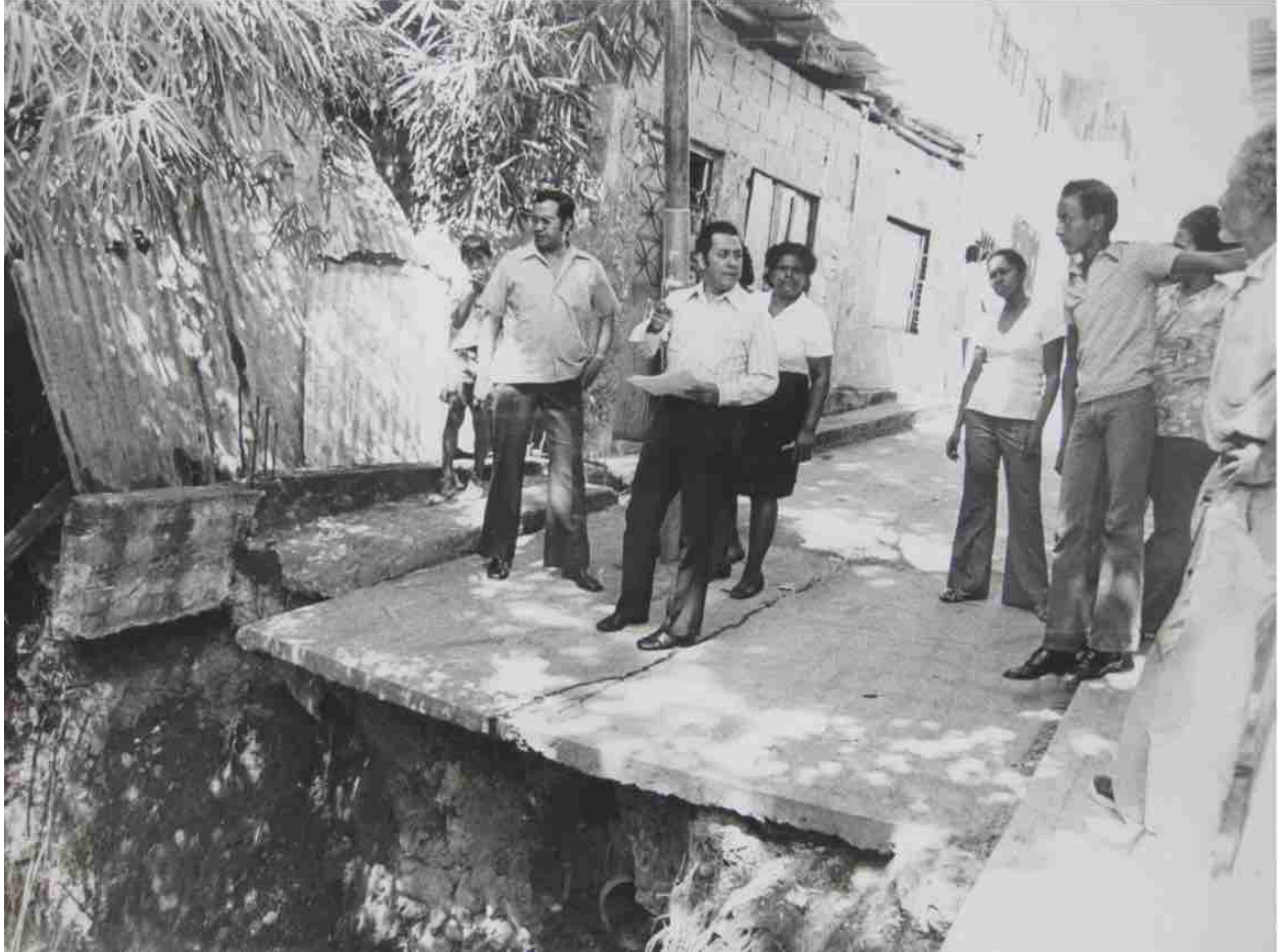
Plate 4.3. Municipal council member Francisco Olivio (Acción Democrática) inspects the flood damage to a retaining wall, street, and nearby buildings in Barrio 24 de Julio, Parroquia La Pastora, caused by a leaky pipe (1974)
