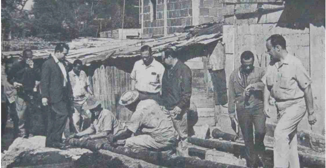
Plate 4.4. A government delegation visits a barrio during a collective work drive ( cayapa ) to install sewage lines, in which relatively few residents participated (1966)
