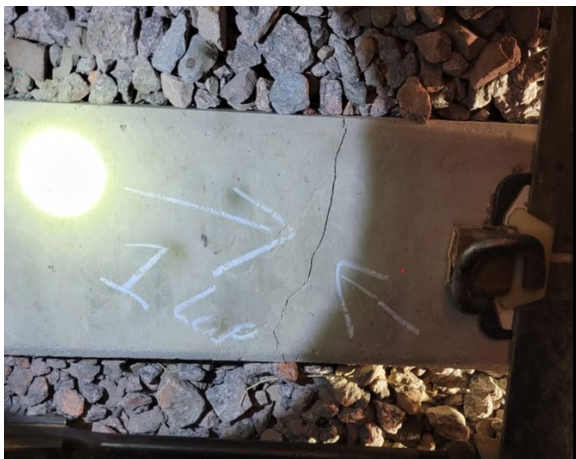
(c) Crack after first lap
