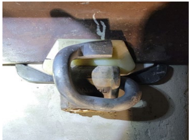
(f) Insulator crack
