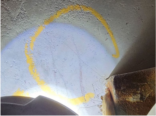
(a) Hairline crack around rail seat
