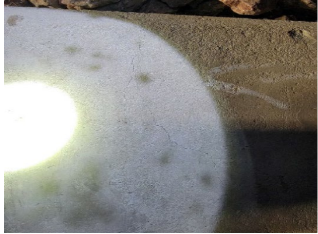
(b) Hairline crack in tie center
