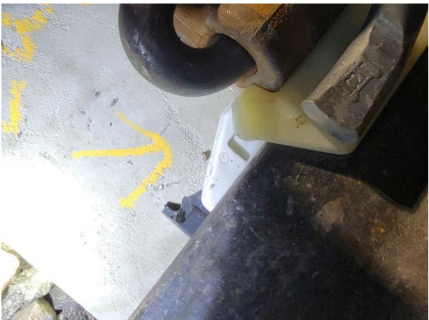
(e) Tie pad breakage
