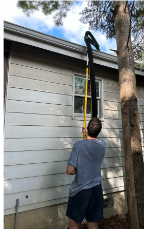
Image 1.4 Team member Max Mancini cleaning the gutters at Professor Ashton-Miller's house using the Gutter Viper.
