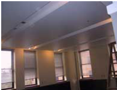
Figure 26: Installed Radiant Panels at S.T. Dana Building
