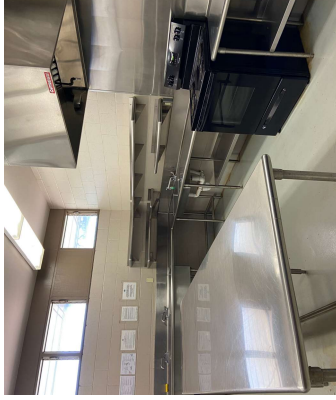
Large Kitchen (stainless steel, grease trap)
