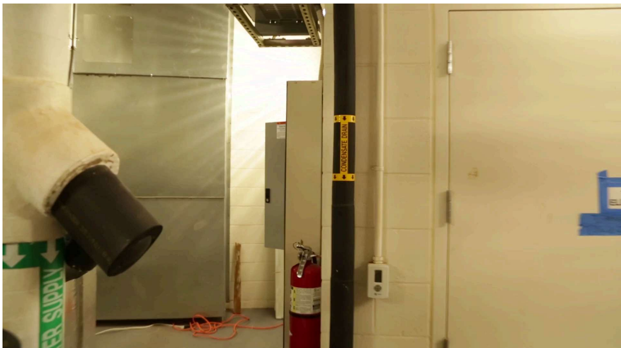
Photo 8. Condensate Drain Pipe . Source: Condensate Drain. University of Hawai'i Sea Grant. (2019). Water Reuse – Hawai'i Sea Grant . Hawai'i Sea Grant. Retrieved March 26, 2024, from https://seagrant.soest.hawaii.edu/water-reuse/
