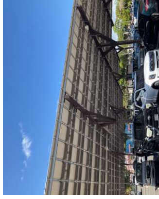
Solar Panels in Parking Lot
