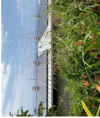
Roof Solar Panels
