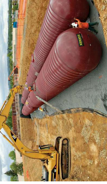
WATER STORAGE TANKS
