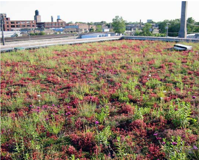
Figure 3.19: A greenroof reduces the building's energy consumption and reduces runoff from the building (CCGT).
