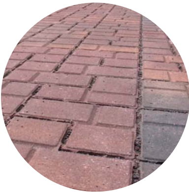
107. Interlocking Permeable Pavers Unilock
