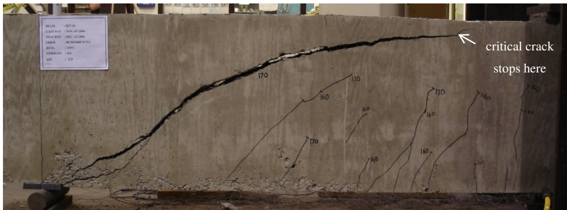
Fig. 4-105: Crack pattern after failure – Beam B27-1b
