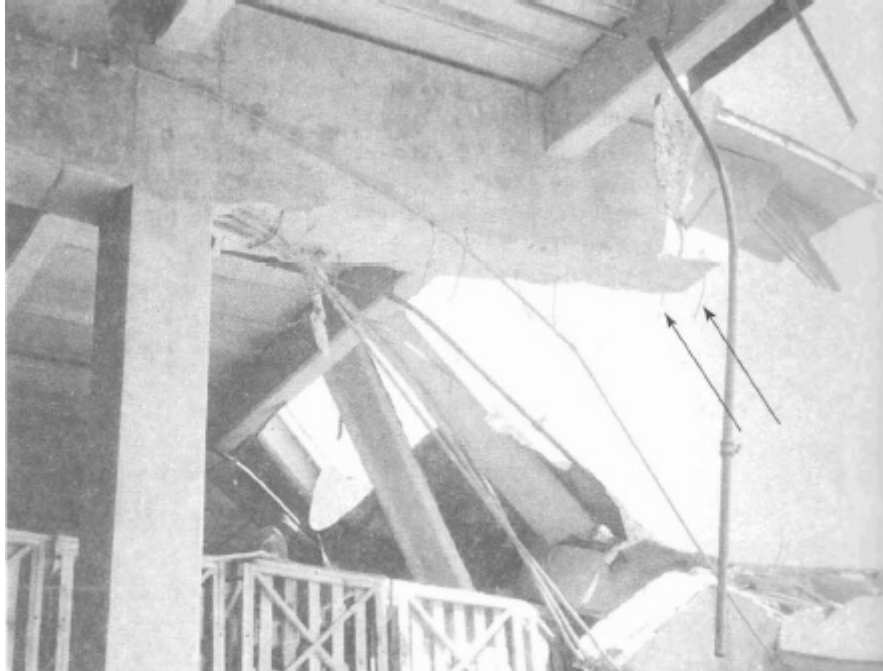
Fig. 1-1: Shear failure of reinforced concrete beams in the U.S. Air Force Warehouse (from Wight and MacGregor, 2009)
