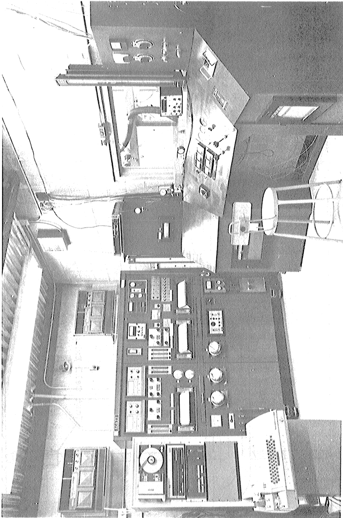
Figure 3.2 Engine Control Room
