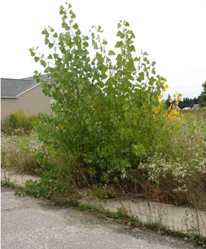
Figure 6: Quaking Aspen grows through a curb on site
